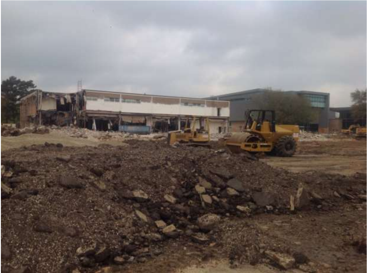
Looking toward the new library from the southeast corner of the parking lot.
