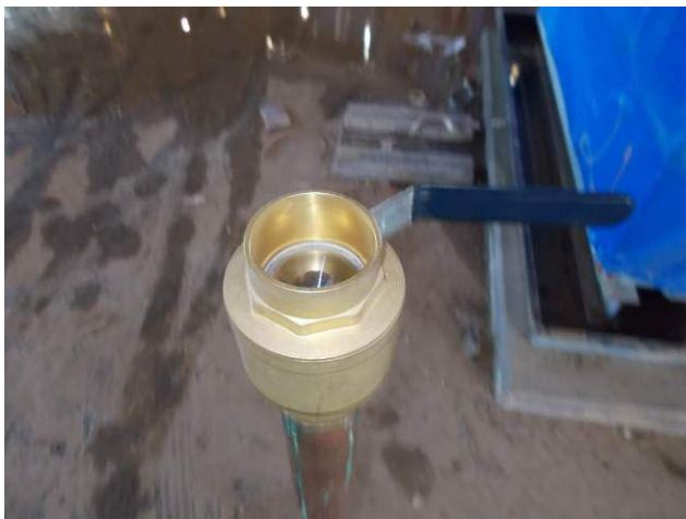
Protect open valve.
