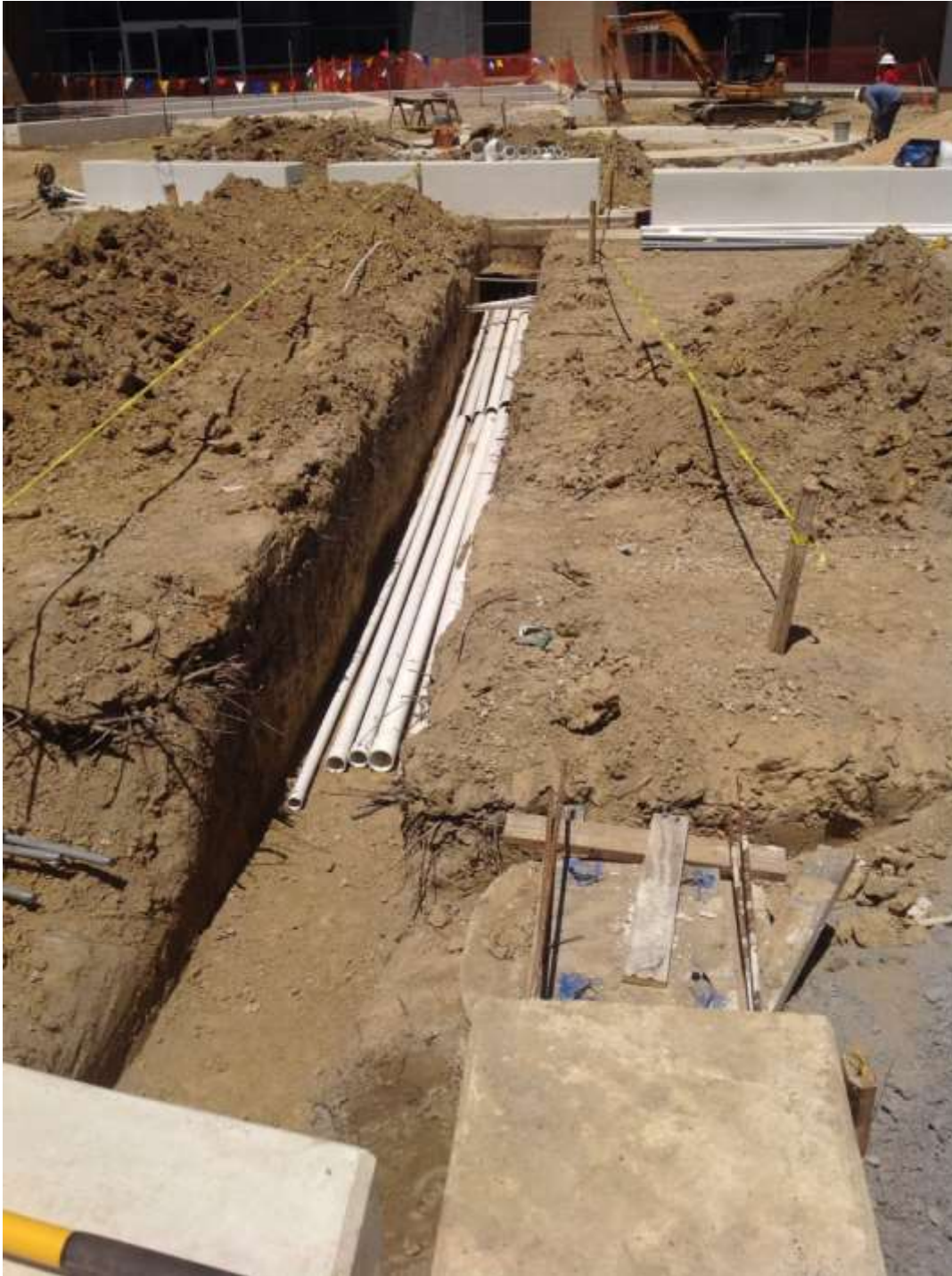
Looking toward the Splash Pad at its plumbing lines
